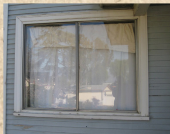
Aluminum sliding window incompatible with Victorian architecture
