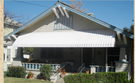
Inappropriate aluminum awning and handrail on Craftsman bungalow
