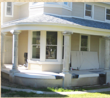
Replacement of decorative turned wood columns with incompatible cast stone columns
