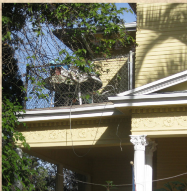
Inappropriate chain link fence on Victorian deck
