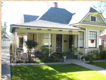
Replacement of decorative classical columns with incompatible tube steel columns
