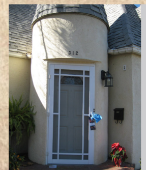
Incompatible prairie-style screen door in whimsical Normandy style cottage.
