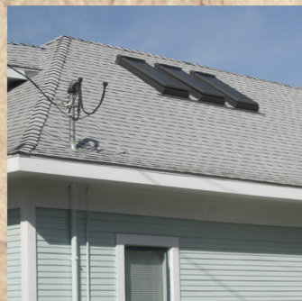
Roof Windows (skylights) are inappropriate to Victorian architecture
