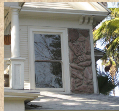
Inappropriate faux stone veneer applied to Victorian edifice
