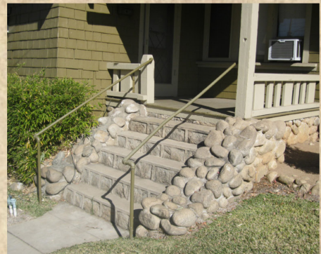
Incompatible pipe hand rail on Craftsman bungalow
