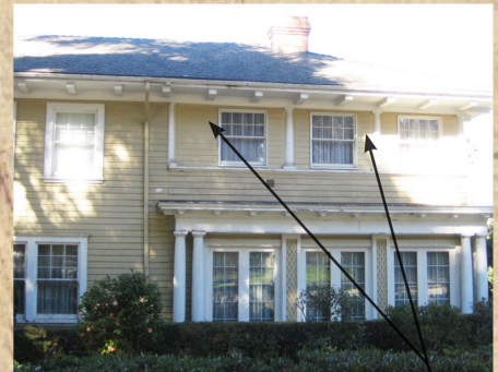
Inappropriate porch infill. Note incompatible shingles and vinyl window in addition.
