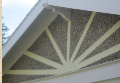
Inappropriate cement infill of decorative wood fan pattern on Craftsman bungalow
