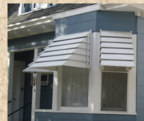
Incompatible aluminum awnings on Victorian residence
