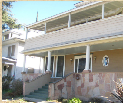
Inappropriate stone cladding applied to first story porch wall
